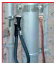
Fence and Gate Jumper Assemblies
