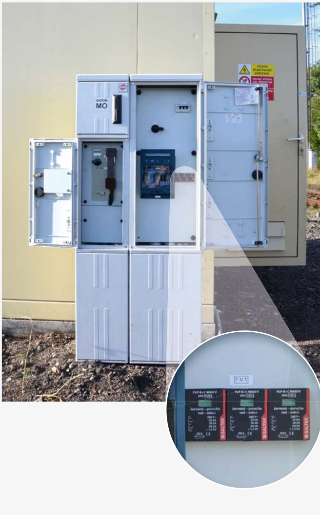
Fig. 2 View to power distribution box of signalling system with installed SPD Type 1 and 2 FLP-B+C MAXI V/3
